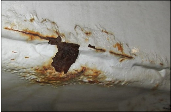
Severe rust that needs further examination
